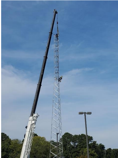
New 120' Communications Tower
