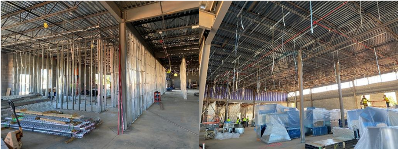
Figure 2: Overhead conduits and interior framing in progress; HVAC ductwork installation to begin soon
