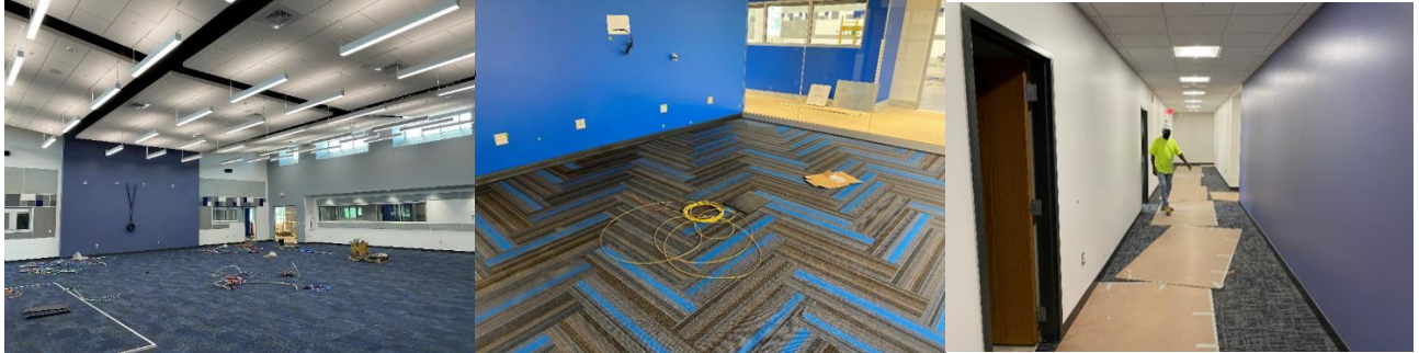
Figure 2: Carpet and sound panels installed in 911 and EOC and other facility areas
