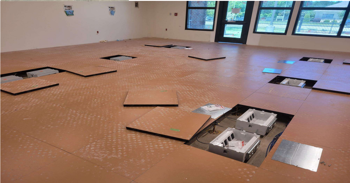
Electrical under the raised floor
