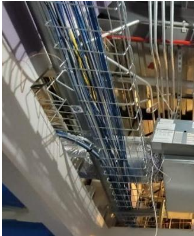
Figure 3: Structured / low voltage cabling installation
