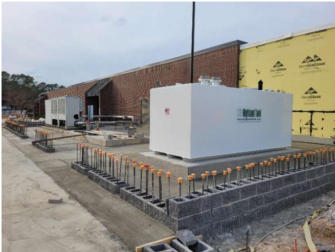
Mechanical yard and fuel tank
